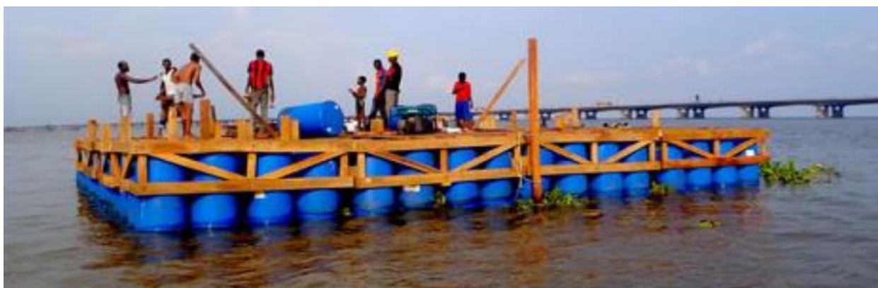
Figure 8: Base of the building during construction of the Floating School. Source: Amy Frearson, Dezeen Magazine. (Available online: https://www.dezeen.com/2014/03/25/makoko-floating-school-nigeria-nle/ )
